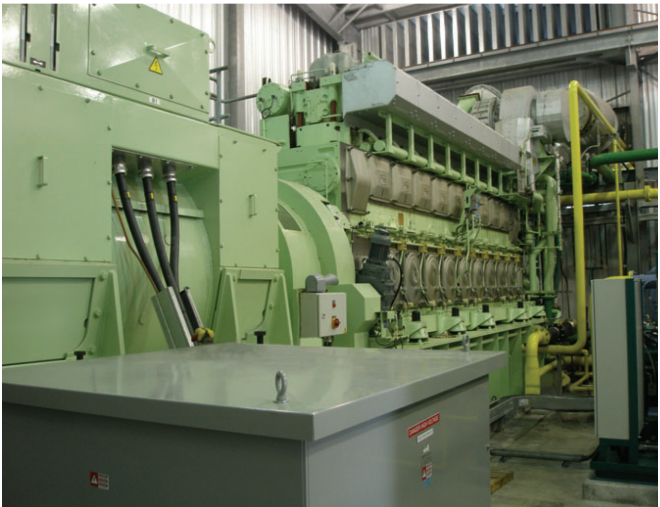
Typical power generating set
